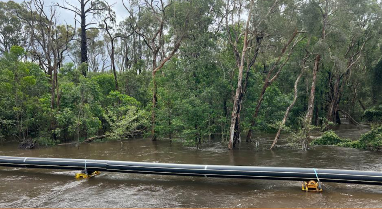
Flooded pipeline alignment in Kawana Forest Bushland Reserve
