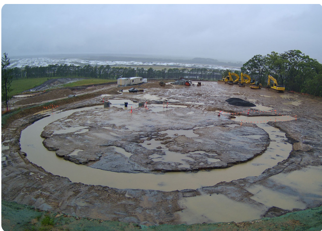
The foundations at the Aura Reservoir construction site resembled a moat after a heavy downpour.
