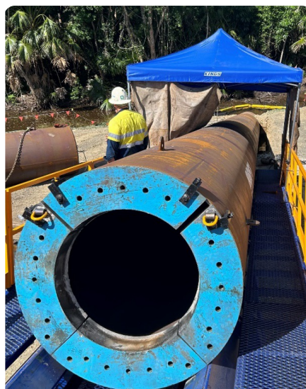
Enveloper casing at Kawana Wastewater Treatment Plant to prevent uncontrolled fluid release
