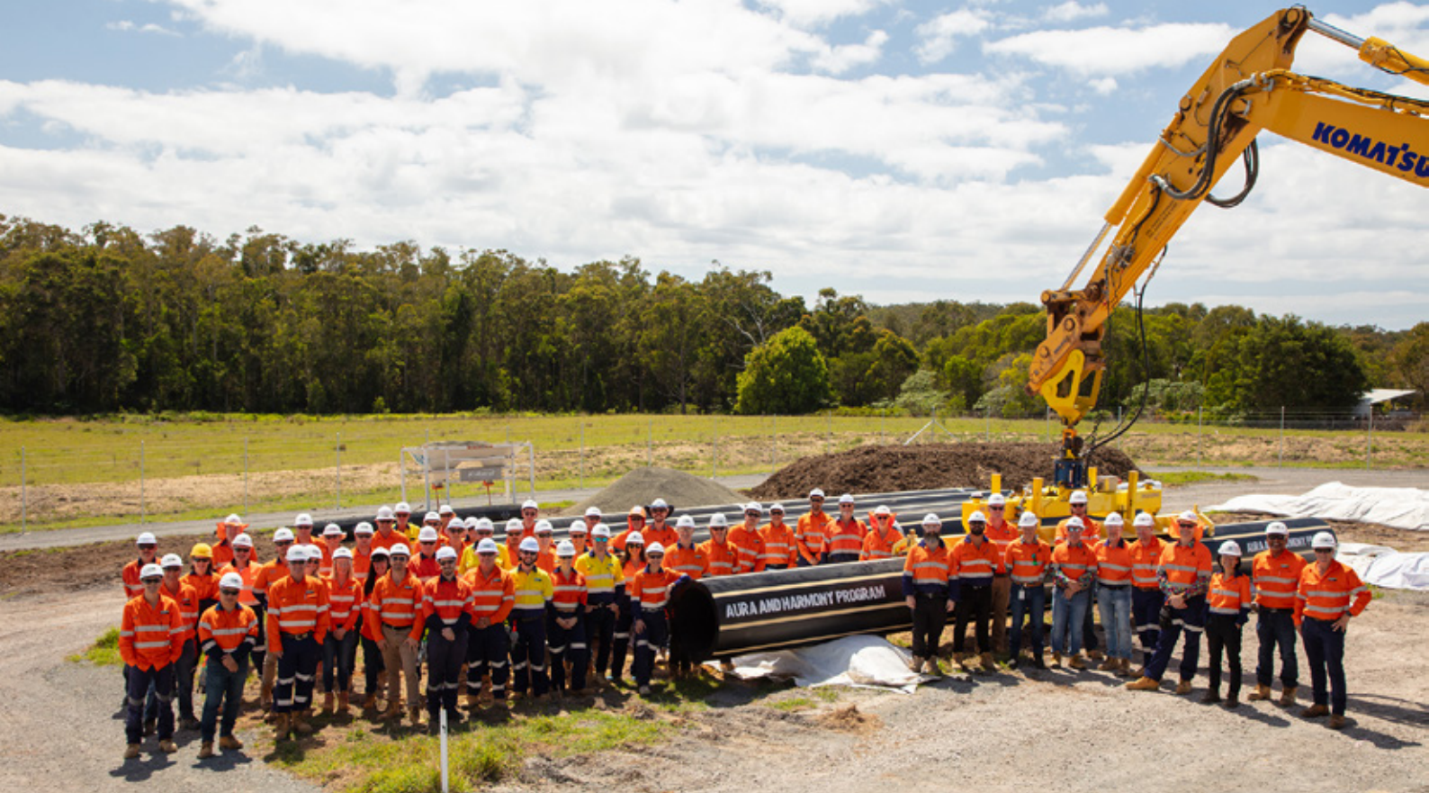
It's a pipe party! The Aura and Harmony Program team celebrating the arrival of the first pieces of pipe at the construction site office in Meridan Plains.
