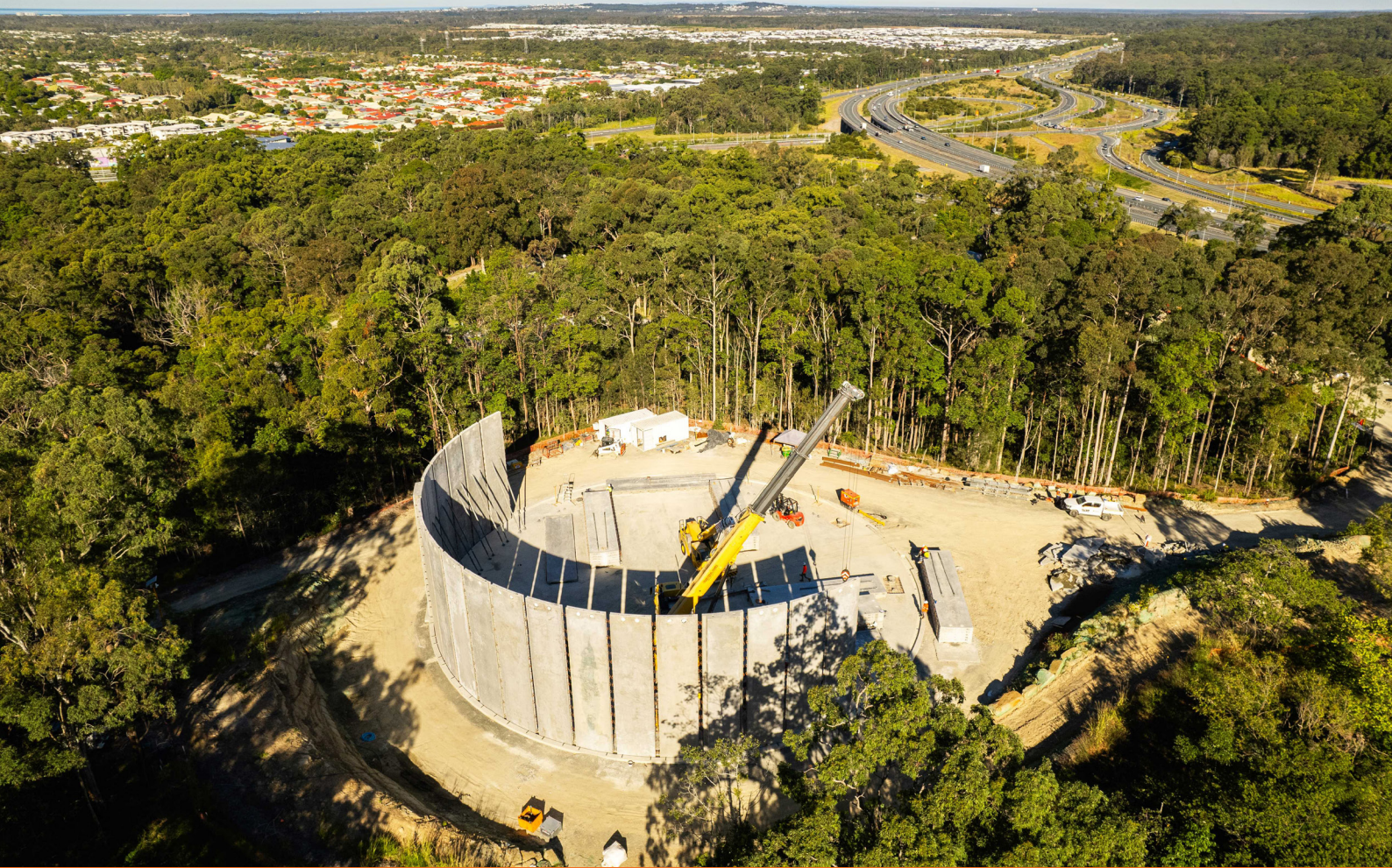
Tanawha Reservoir is on time and on budget to supply safe and reliable water to the growing Harmony community (in the background).
