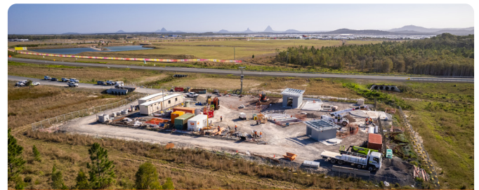
Aura Wastewater Project's new wastewater pump station with Aura development in the background.
