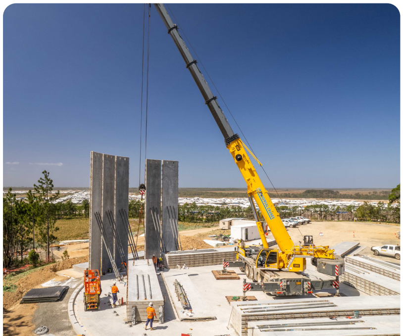
New Aura water reservoir takes shape on the western side of the Bruce Highway, across the road from the Aura development.
